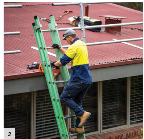
1-3. A range of examples on correct use of ladders while working at height.
